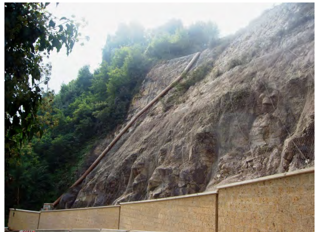
Figure 5a Orvieto (Terni, central Italy), road “SP111 della Badia” Situation of the slope in December 2004, before intervention
