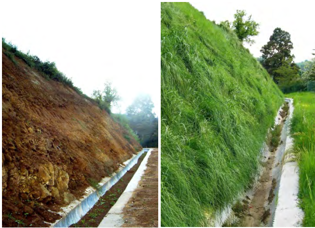
a) clogged drains
