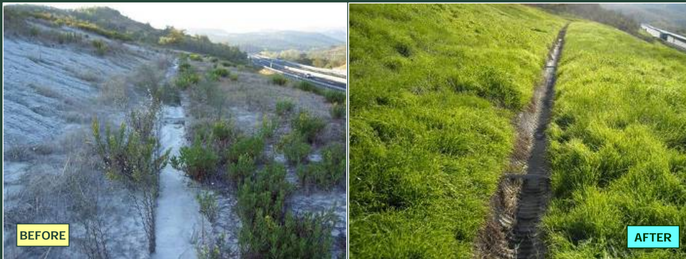
Perfectly clean ditches at the base of a PRATI ARMATI® installation (center Italy, Motorway A1)
